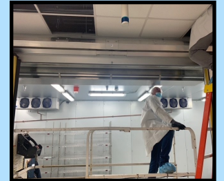
10' Air Curtain in Cooler
